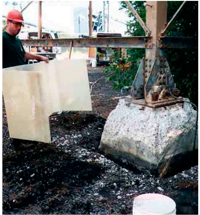
Foundation prepared and excavated; FX-70® jacket installed below ground level for additional protection
