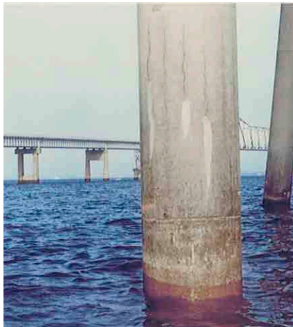
Example of pile "scour"
