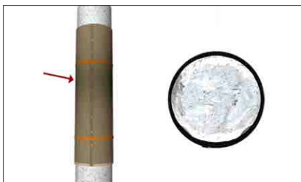
Piles with \leq 25\% section loss, fill remaining void in jacket with FX-70-6MP™. Piles with > 25\% section loss, fill void with FX-225 Underwater Grout, leaving 100 mm open at top of jacket (allow to cure overnight); fill remaining 100 mm with FX-70-6MP™ (allow to cure overnight).
