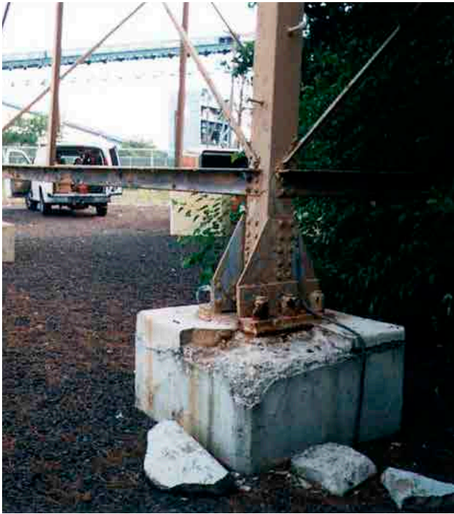
Severe damage to concrete foundation
