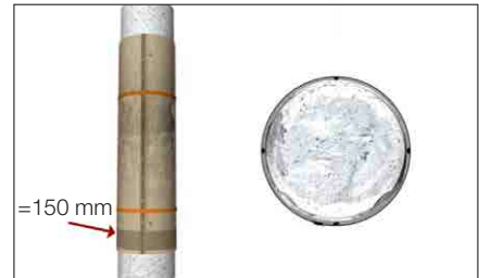
Install 150 mm of FX-70-6MP™ Marine Epoxy Grout to create bottom seal; allow grout to cure overnight.
