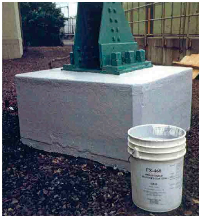
Repair completed with FX-70-6MP™ Multi-Purpose Marine Epoxy Grout as the bottom and top seal material. Coating system is used as a final finish on the outside of the FX-70® jacket.
