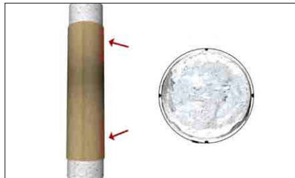
Insert the tongue into the locking groove of the jacket and position it leaving 460-610 mm of jacket above and below the damaged area.
